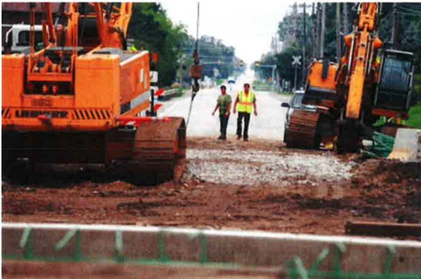
Construction continues Thursday on a bridge off Winn Road north of Route 12 in Spring Grove. The Winn Road bridge is one of several currently being replaced across McHenry County. (Mike Greene – mgreene@shawmedia.com )
