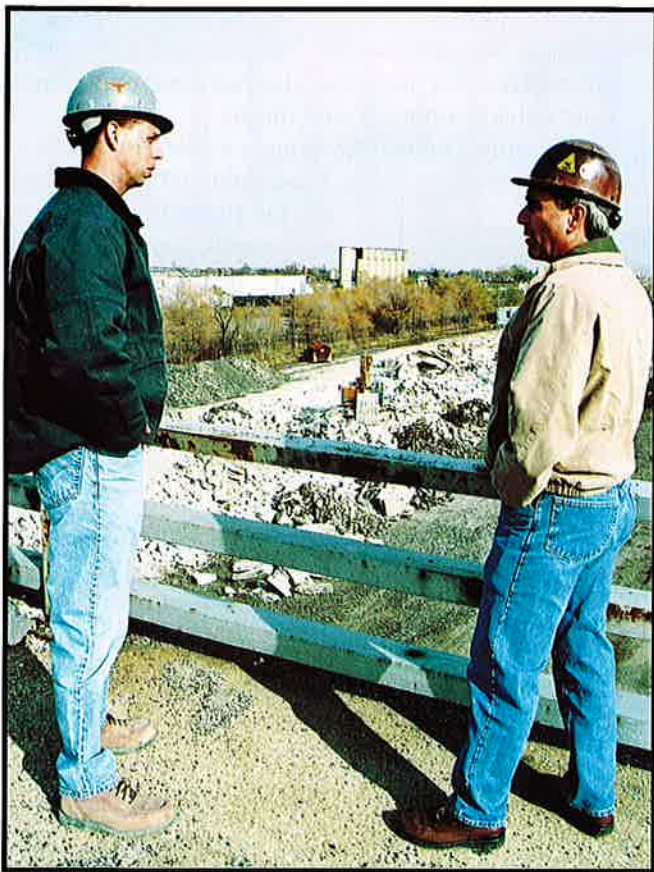
Project Manager Mike Paine, left, and Doug Stuart confer over demolition of the Central Avenue Viaduct in Chicago.
