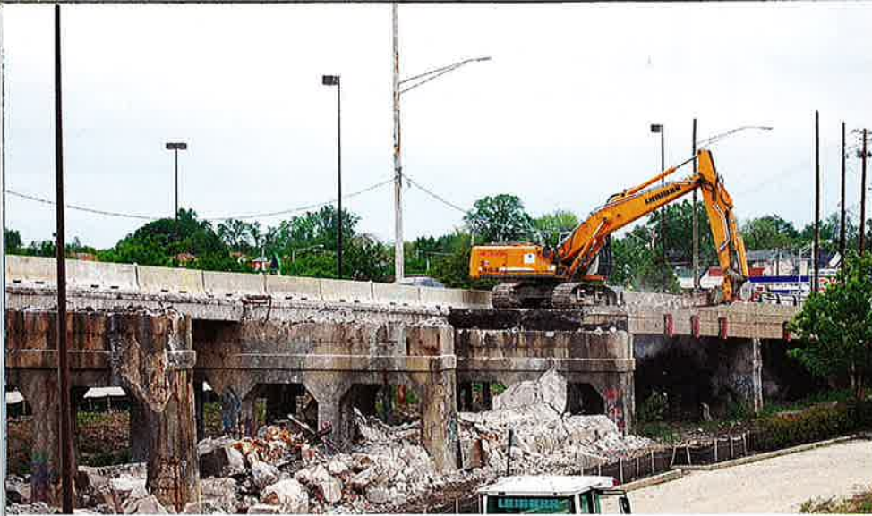
Dunnet Bay does its own demolition work utilizing the Liebherr excavators' versatility to use hammers, shears or grapples or other attachments. The machine's stability makes it possible to meet challenging jobs.
