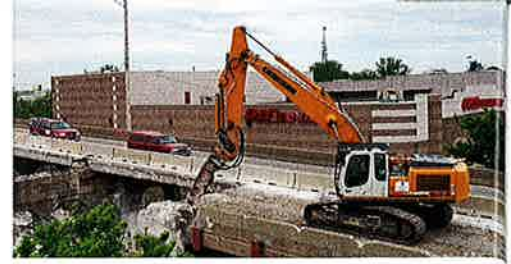
According to Doug Stuart, the operators really like the Liebherr excavators because they are operator-friendly, very responsive and comfortable.
