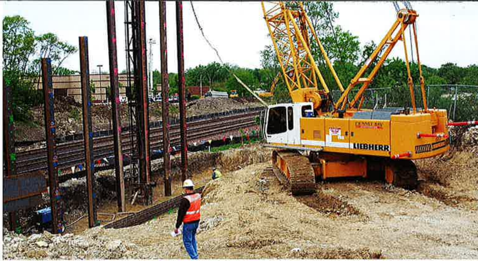
Dunnet Bay uses the Liebherr crawler cranes for hoisting as well as driving sheeting for footing and foundation work. According to Doug Stuart, owner and partner, the company depends on the cranes because of the amount of bridge work that they do.
