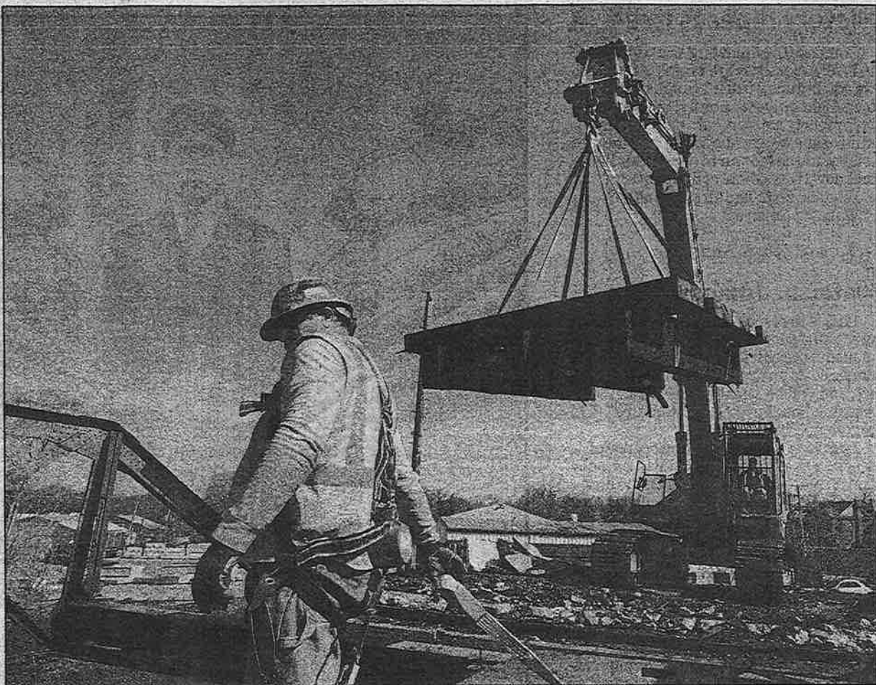
A crane lifts a piece of the timber deck cut by laborer Frank Ortiz, foreground. Demolition of the Wesley Street-Manchester Road bridge was completed recently. CHUCK BERMAN/TRIBUNE PHOTO
