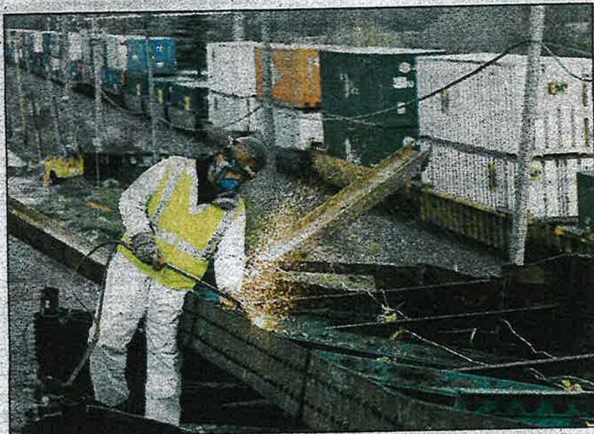
R.J. Hopper uses a torch to cut the trusses of the bridge at Wesley Street and Manchester Road in Wheaton. The bridge was closed to traffic in November.
